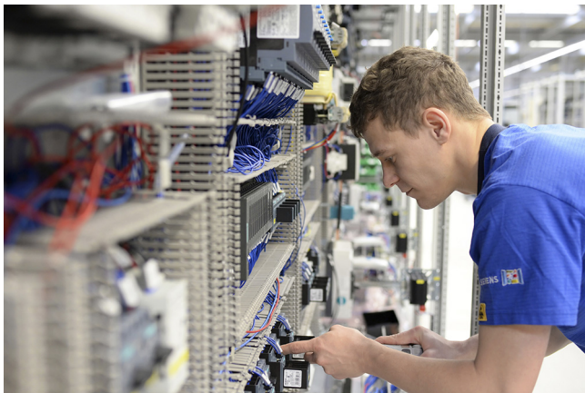
WKC - Control cabinet wiring
